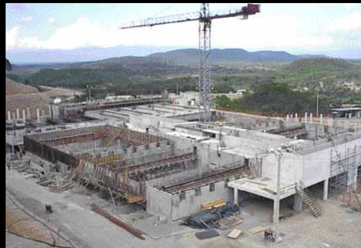
Mao Point Wastewater Treatment Plant, Dominican Republic
